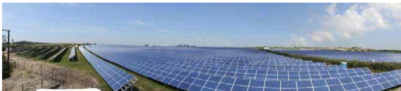
Solar PV facility adjacent to Saarbruecken airport
